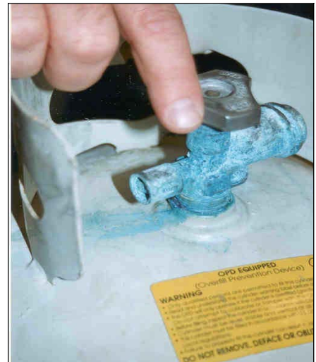
Blue valve means danger!
